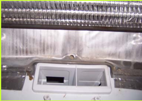
Drain hole in back of freezer
