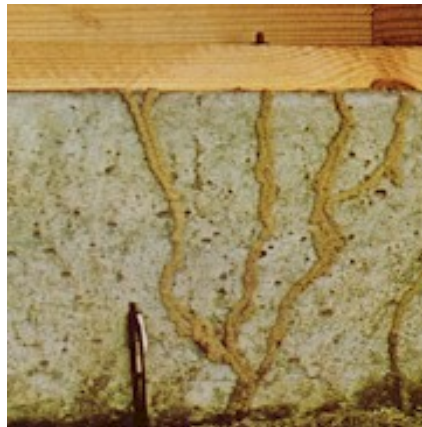
Termite tunnels along foundation
