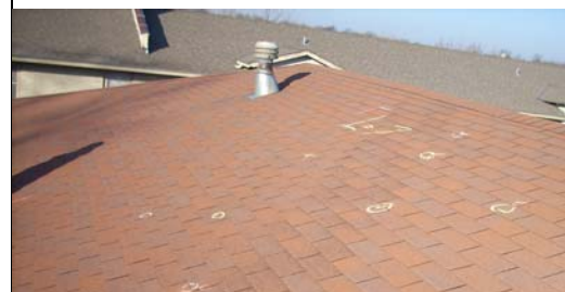
Eight hail hits in 10 ft. x 10 ft. area
