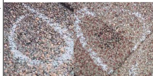
Hail damage to shingles
